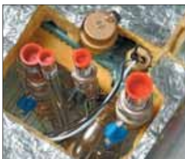
Flow, Return, Hot and Cold valved connections
